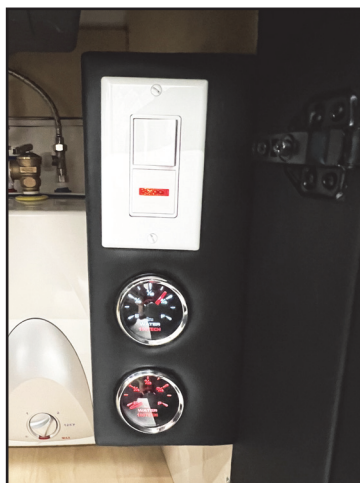
Water Tank Gauges
