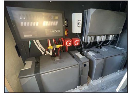
10,000 Watt Power System
