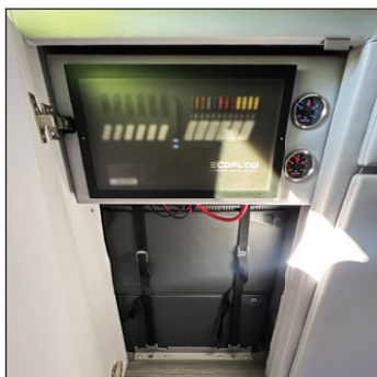
Power Hub & Batteries
