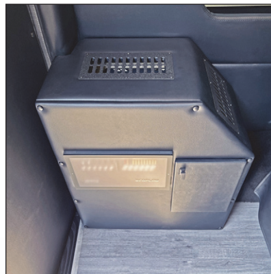
Power System with 5,000W Lithium Battery
