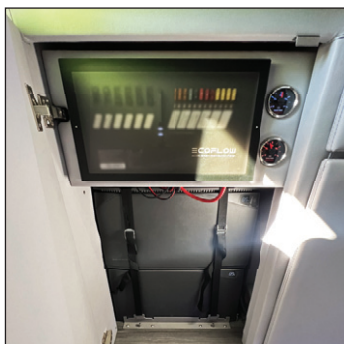
Power Hub & Batteries
