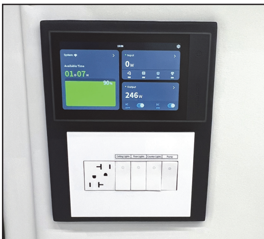
Power System Controller
