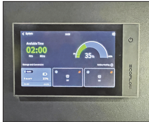
Power System Controller
