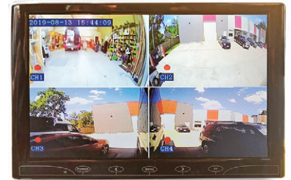
Four-Camera Security System
